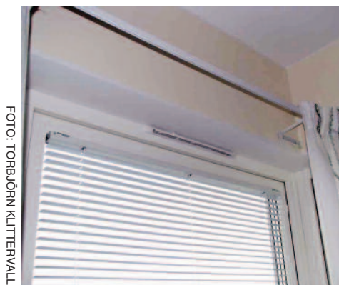
Figur 6: Spaltventiler ger ofta dragproblem.
